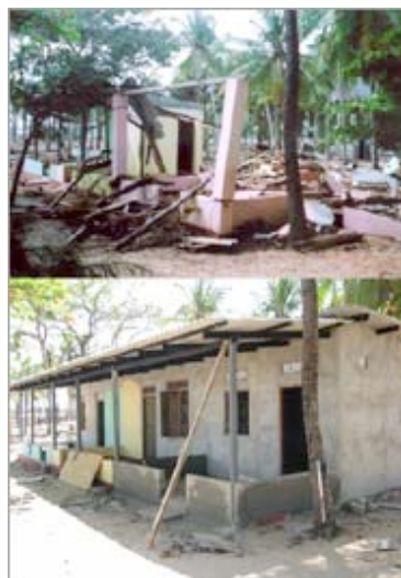
Wreckage of the French Garden Pragash Guest House a few days after the tsunami and the repair work completed at the end of February. Before picture courtesy of Raj Pragash.
