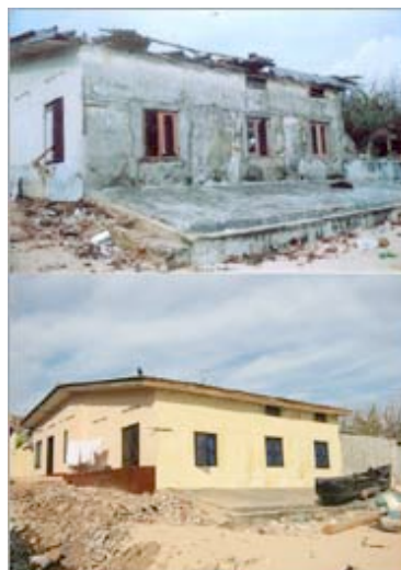
Damage at the Dyke Corner Inn in Trincomalee a few days after the tsunami and the repair work completed at the end of February. Before picture courtesy of Dyke Corner Inn.
