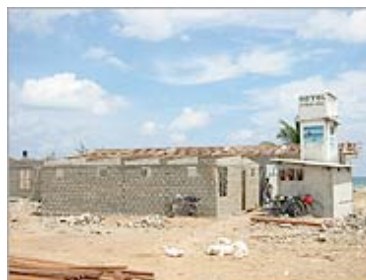
Work continues on the Coral Bay Hotel in Nilavelli. What's the future of such small guesthouses?
